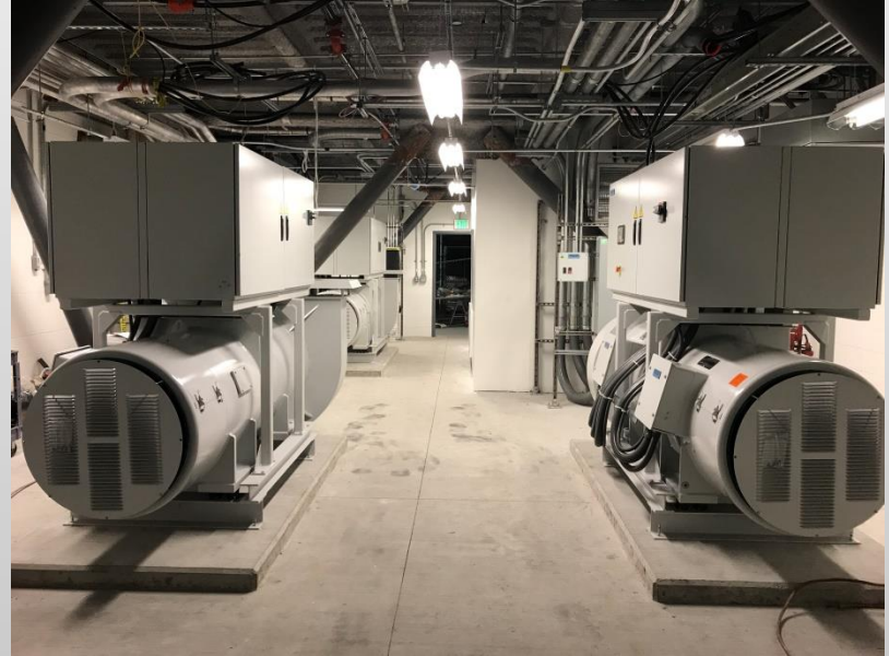
Gate Utility Improvements – Motor Generators
